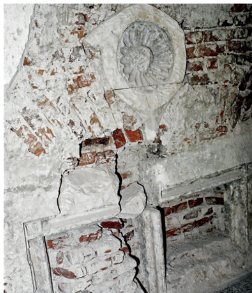
Češki prozor na istočnom zidu zapadnog tornja Czech window on the eastern wall of the western tower
