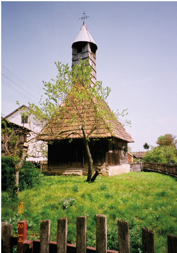
1. Zapadno pročelje kapele prije građevinske sanacije (fototeka HRZ-a, inv. br. I 130121, snimila J. Bartoniček, 1994.) West front of the chapel before the construction repair (Croatian Conservation Institute Photo Archive, inv. no. I 130121, photo by J. Bartoniček, 1994)
