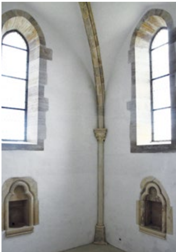
13. Gora, crkva Uznesenja BDM, pogled na niše u svetištu nakon završetka radova (snimio D. Miletić). Gora, Church of the Assumption of the B. V. Mary, view of the niches in the sanctuary after conservation (photo by D. Miletić)
