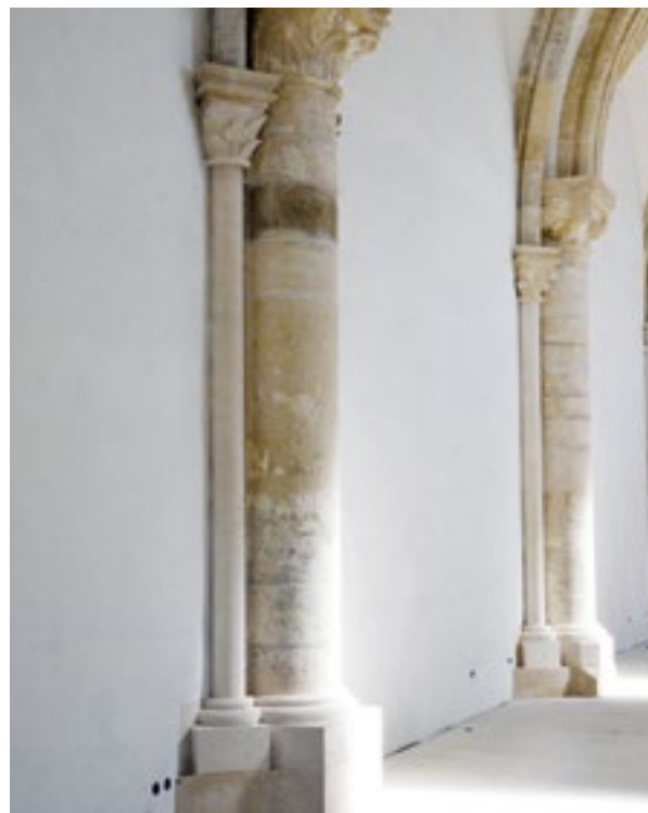
21. Gora, crkva Uznesenja BDM, unutrašnjost, pogled sa zapada na južni zid nakon rekonstrukcije (snimio D. Miletić). Gora, Church of the Assumption of the B. V. Mary, interior, view from the west of the southern wall, after reconstruction (photo by D. Miletić)
