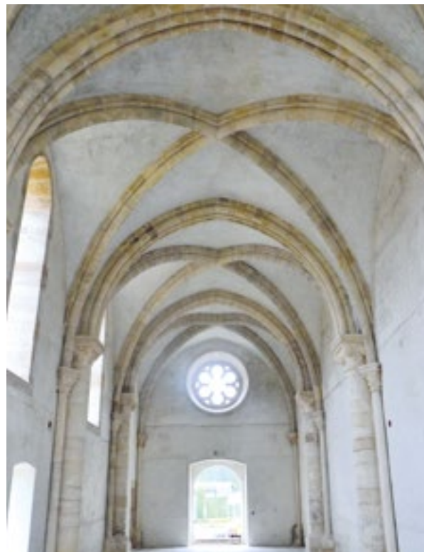
19. Gora, crkva Uznesenja BDM, unutrašnjost, pogled prema zapadu nakon rekonstrukcije (snimio D. Miletić). Gora, Church of the Assumption of the B. V. Mary, interior, view of the west after reconstruction (photo by D. Miletić)
