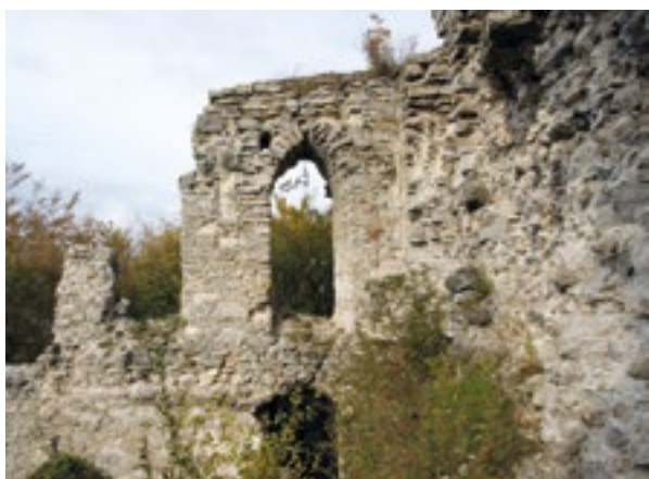
7. Tehnika zidanja pločastim kamenjem na sjevernom zidu kapele (fototeka HRZ-a, snimio V. Madiraca, 2008.). Flat stone masonry on the northern wall of the chapel (Croatian Conservation Institute Photo Archive, photo by V. Madiraca)
