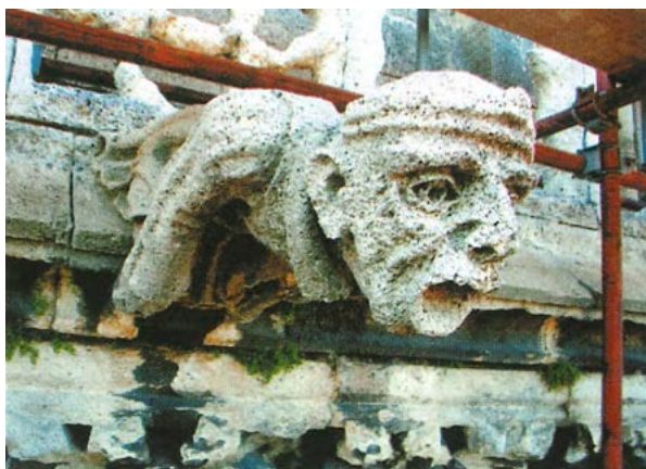
5. Stara i oštećena rigalica na sjevernom tornju katedrale, sačuvana in situ (izvor: RUKAVINA, 2004, 20) Old, damaged waterspout on the north tower of the cathedral, preserved in situ (from: RUKAVINA, 2004, 20)
