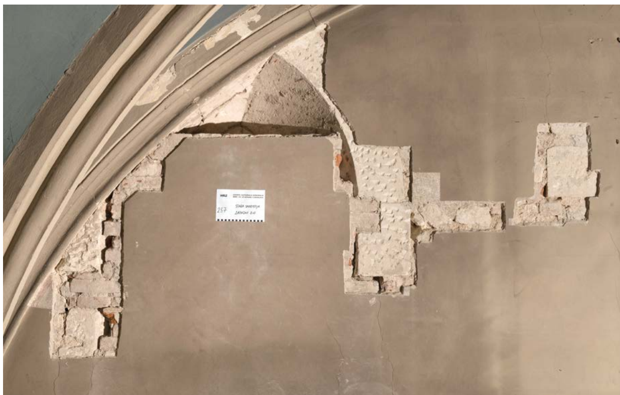
15b. Sonda 257, otkriveni srednjovjekovni prozor na zapadnom zidu sakristije kojem je izvorno tjeme preoblikovano rebrom svoda iz vremena biskupa Timoteja (arhiva HRZ-a, sondirao: M. Deak, snimka: K. Gavrilica, 2023.) Probe 257, a newly-discovered medieval window in the western wall of the sacristy, whose original top was reshaped with a rib of the vault from the time of Bishop Timotheus (HRZ Archive; probe: M. Deak; photo: K. Gavrilica, 2023)
