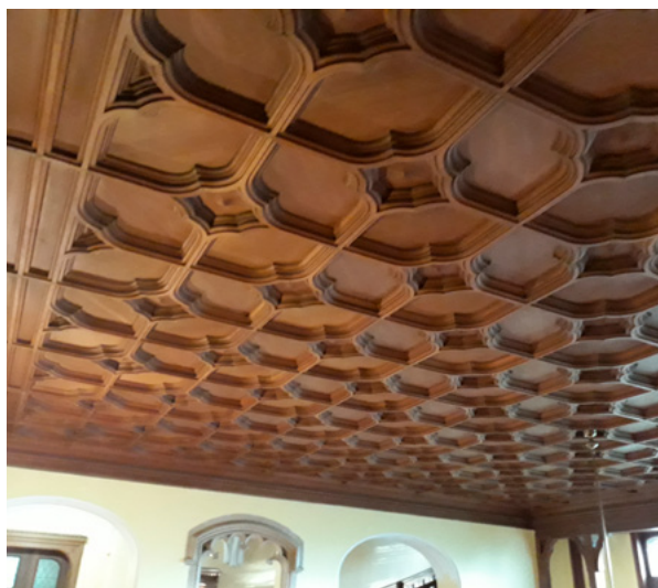
11. Drveni strop u dvorcu Hilleprand-Mailáth u Donjem Miholjcu, 1903. – 1907. (snimio D. Trcović, 2018.) Wooden Ceiling in the Hilleprand-Mailáth Castle in Donji Miholjac, 1903–1907 (D. Trcović, 2018)
