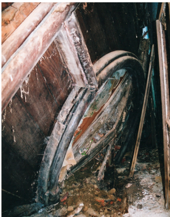
4. Jedan od medaljona nakon urušavanja krovišta i stropa dvorca (fototeka MK RH, KO Zagreb, snimio N. Bradić, 2003.) One of the medallions after the collapse of the manor house roof and ceiling (Ministry of Culture of the Republic of Croatia, Conservation Department in Zagreb Photo Archive; N. Bradić, 2003)
