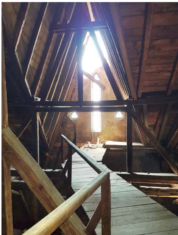
2. Oštećeni pokrov i drvena konstrukcija krovica te kameni zabatni zid najzapadnije krovne kućice – wimperga , pogled iz krovšta (fototeka GZZSKP-a, 2020.) Damaged cover and wooden structure of the roof and the stone gable wall of the westernmost crowning ( wimperg ), view from the roof (GZZSKP Photo Archive, 2020)
