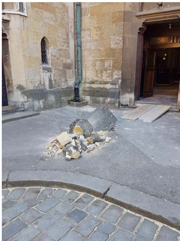
3. Kameni element križne ruže srušen s vrha timpanona krovne kućice na sjevernoj strani ispred ulaza u sakristiju (fototeka GZZSKP-a, 2020.) Stone element that had fallen from the top of the pediment of the crowning on the north side in front of the entrance to the sacristy (GZZSKP Photo Archive, 2020)
